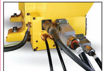
Utility connections at base
